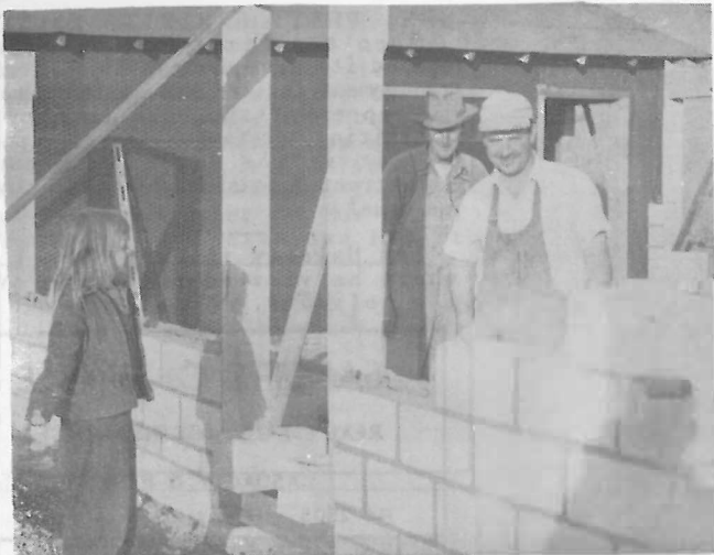
SMALL FRY SHOWS INTEREST IN NEW YOUTH CENTER BUILDING WHERE BOB WOOD AND LONNIE DENNIS LAY BRICKS FOR RESTROOMS AND KITCHEN. - IRVINE PHOTO.
